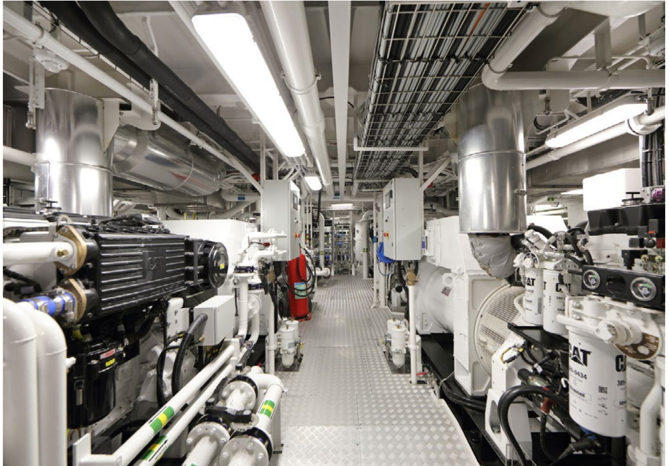
LOWER DECK - ENGINE ROOM
