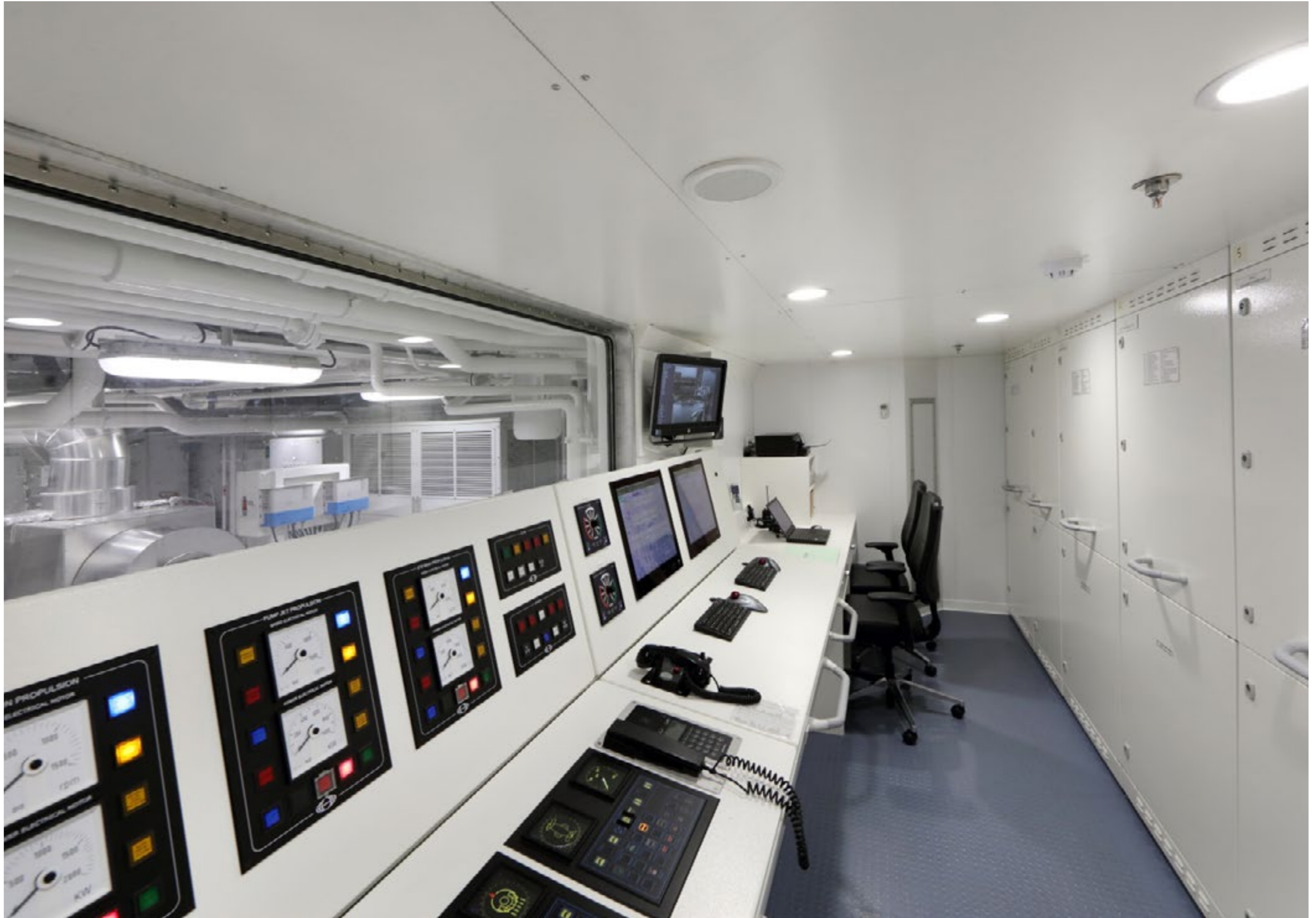
LOWER DECK - CONTROL ROOM
